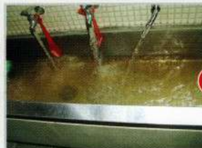
▲取付前の蛇口部の赤水 Before installing (rusty water from the tap).
