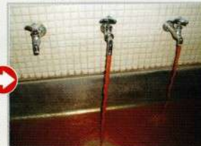
▲取付直後の蛇口部の赤水 After installing (red rusty water from the tap).
