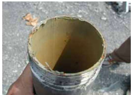
Pipe with Ion Water installed
